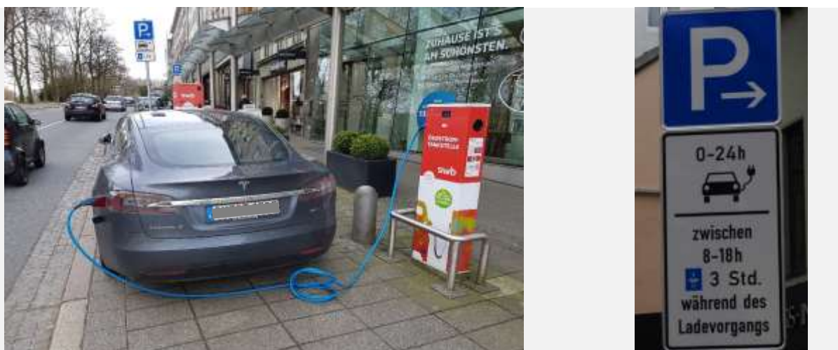
On-street charging infrastructure needs a business case – requiring limited parking/charging time (example: only for e-cars during the charging process, max 3 hours parking between 8:00 and 18:00) (photos: Glotz-Richter)
