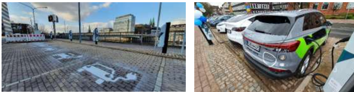
Charging hub in Bremen with six charging points at one grid connection (under construction and in use) (photos: Glotz-Richter)
